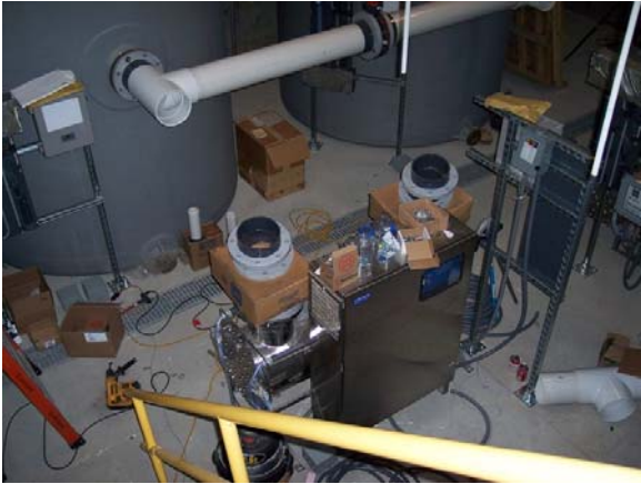
Setting the Ultraviolet Disinfection Units
