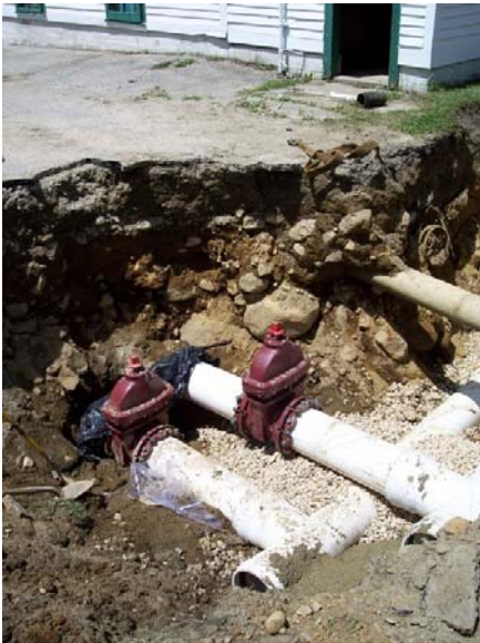
Gate Valves on 12" PVC Water Supply Pipes
