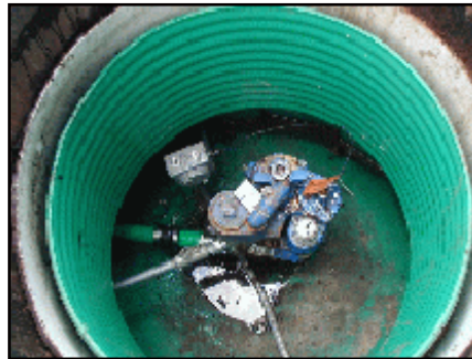
Sample Flexible Piping in a Sump
