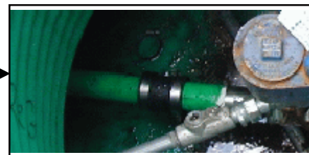
Close-up of Flexible Piping in a Sump
