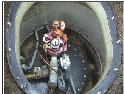
Sample STP Head in a Sump on Top of a Tank
