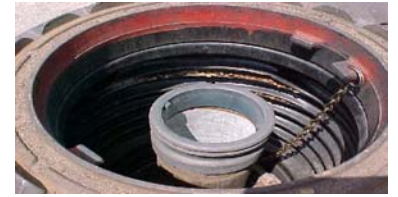
A close-up view of the interior of one of the spill buckets at the Mississippi truck stop. The backfill material is clearly visible through the cracked plastic. Photo courtesy of the Mississippi Department of Environmental Quality.
