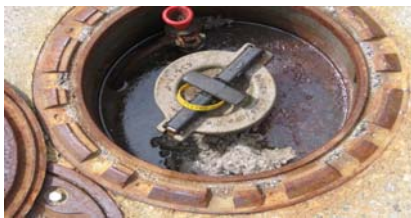
Here is a spill bucket we found in Vermont this past winter – partially filled with road salt!
