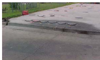
Note the extensive staining surrounding the fill ports at the Mississippi truck stop. Clearly, the delivery drivers were not being as careful to avoid spills as they should have been. Photo courtesy of the Mississippi Department of Environmental Quality
